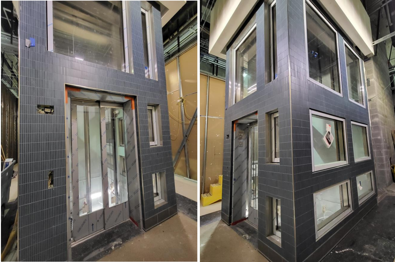
New second elevator
